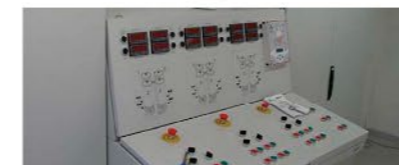
General control board. Tablero de control.
