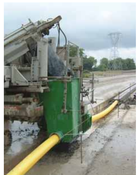
Slotted drain showing inflated tube.
