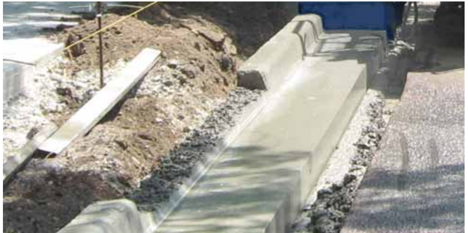
Driveway knives reduce wasted material and labor. Some hand finishing is required.
