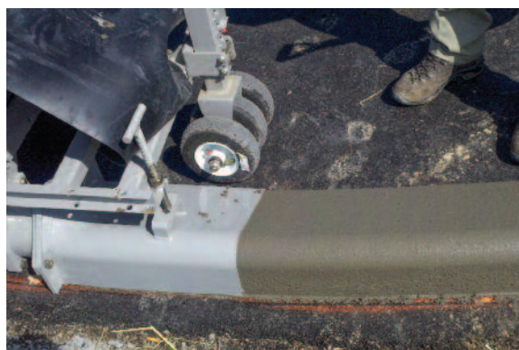
Using a chalk or paint line on the ground as a guide, the operator has a clear view of the path in front of the machine.
